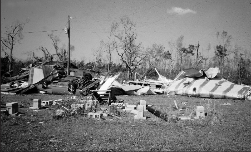
Figure 5-9. A manufactured home that failed during a high-wind event.
