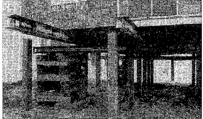
Steel beams are used to lift and support the residence during the relocation process.
