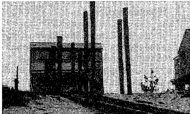
Because driving piles requires heavy machinery, a building being elevated in place may have to be temporarily moved aside and set on cribbing until the driving of piles is complete.
